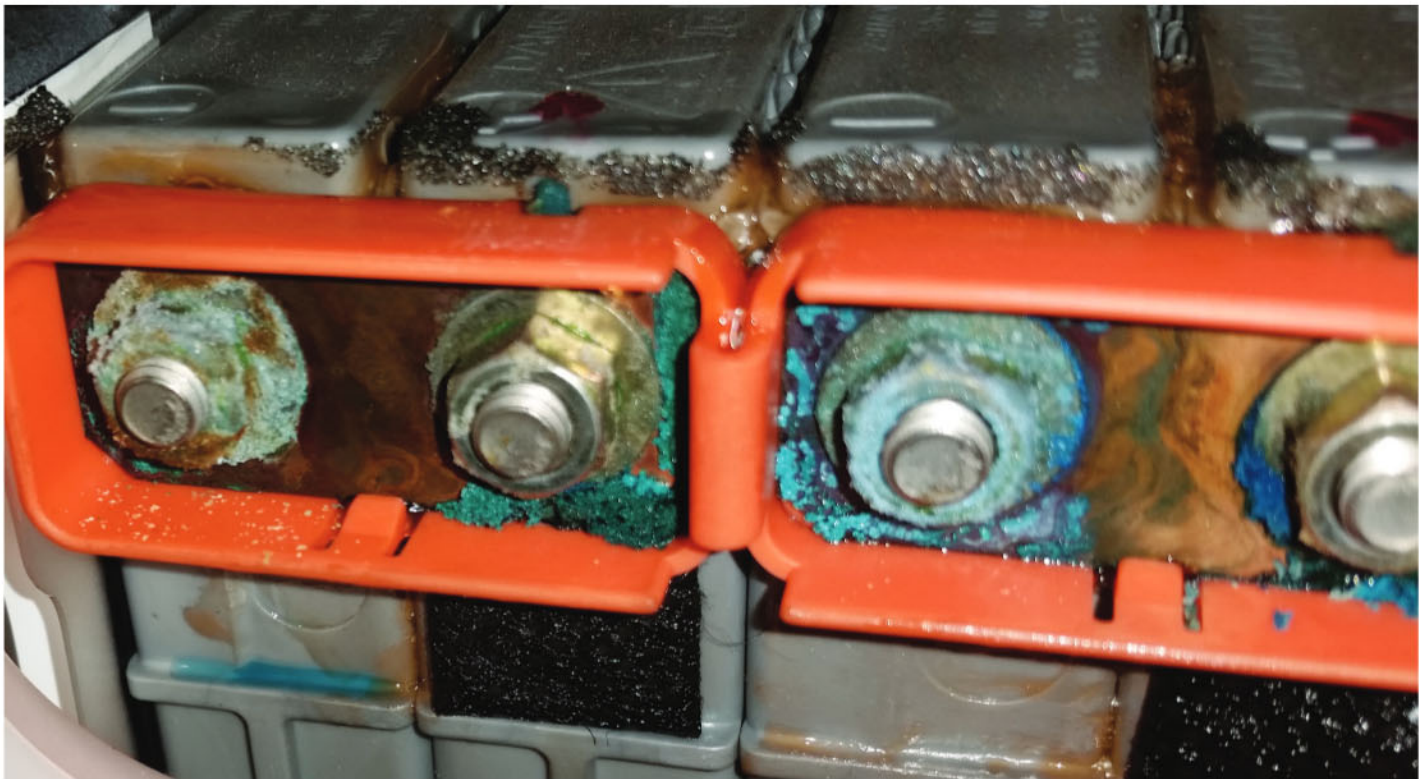
This 18-year-old Prius battery is leaking electrolyte from the battery terminals (note the plug liquid below the first terminal). The foam air dam on the battery cover was soaked in electrolyte and caused a loss of isolation.
